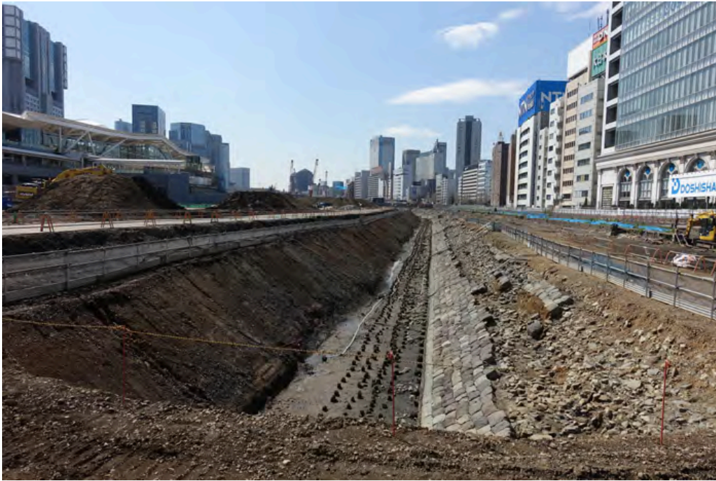
View towards Shinagawa from the northern part of the site. Takanawa Gateway Station is on the left. You can see the linear extension of the well-preserved Chikutei embankment and wooden pile lines in front.
